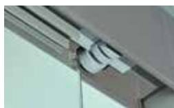
2 Sensors for detector of sash position
